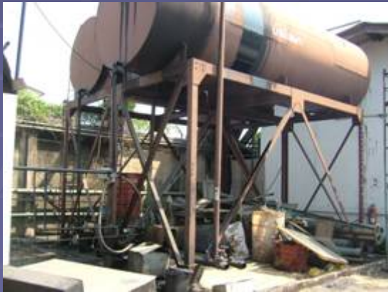
Fuel Oil Storage Tank
